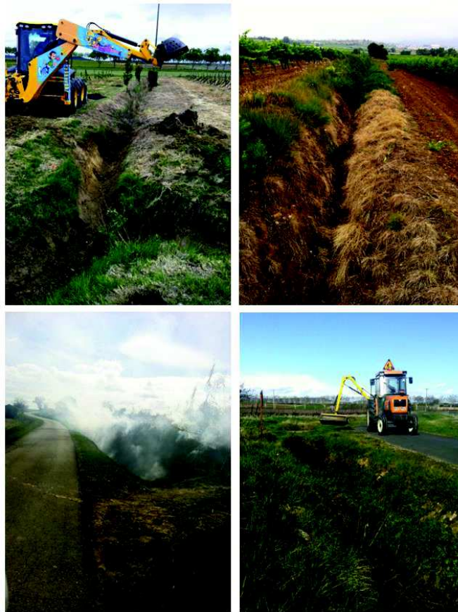
Figure 1.1: Ditch maintenance. Ditch maintenance is a combination and a succession in time of four basic operations namely dredging, mowing, chemical weeding and burning. On top: dredging on the left and chemical weeding on the right. On the bottom: burning on the left and mowing on the right.
